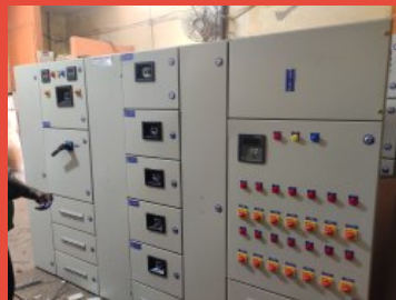
Automatic Power Factor Capacitor Panel
